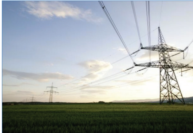
400kV corner mast with OPGW earthwire
