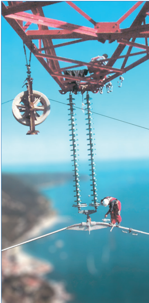
Bosporus Crossing: Double I-insulator string with a saddle type suspension clamp
