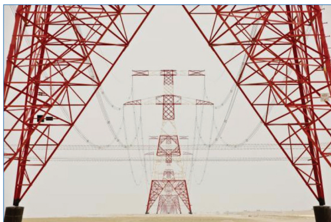
High-voltage line with spacer dampers
